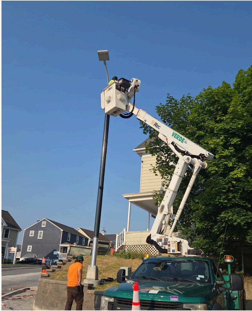
FIELD SERVICE & COMPONENT ACCESS
